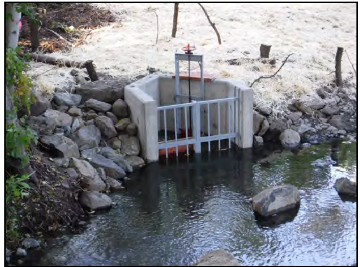
The new efficient irrigation headgate that replaced the Beeson-Robison Dam
