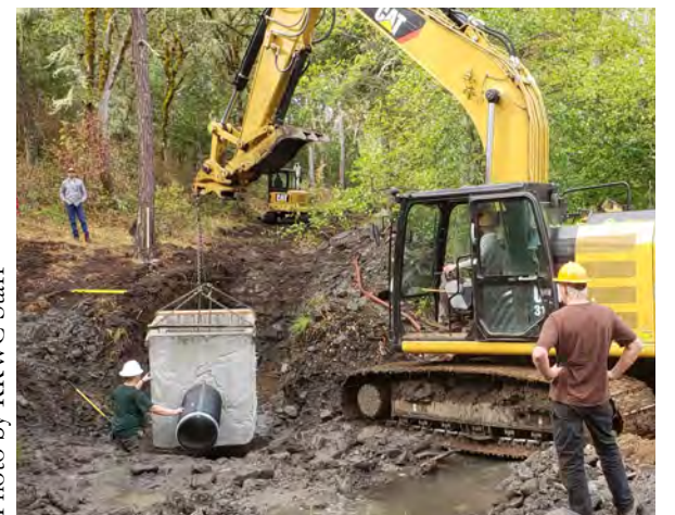
Trask Design and Construction implements Cascade Stream Solutions' design to improve fish passage and irrigation efficiency in Salt Creek.
