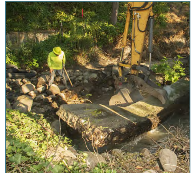
M&M Services implements the design of Cascade Stream Solutions to improve fish passage at the Smith-Myer-Roper diversion site on Ashland Creek
