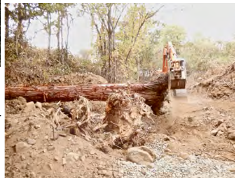
Large wood placement at former dam site during channel regrading (early September 2015).
