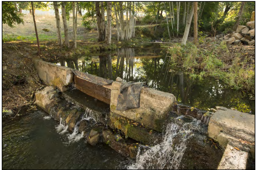
Beeson-Robison dam with flashboards in place prior to removal
