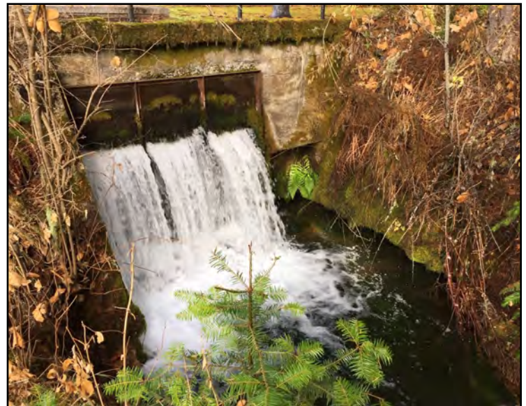
Intake chamber with overflow water at Big Butte Springs
